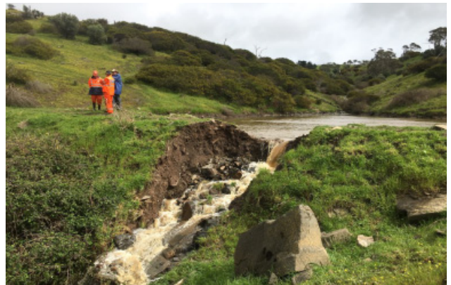
Figure 2: Overtopping dam failure
