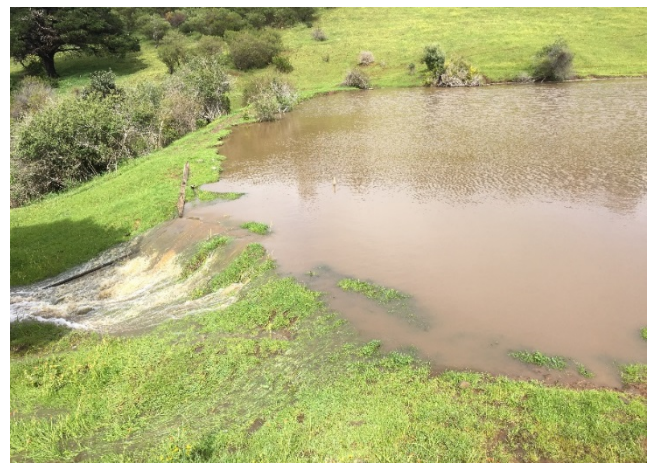
Figure 1: Overtopping of dam at full capacity (prior to failure)
