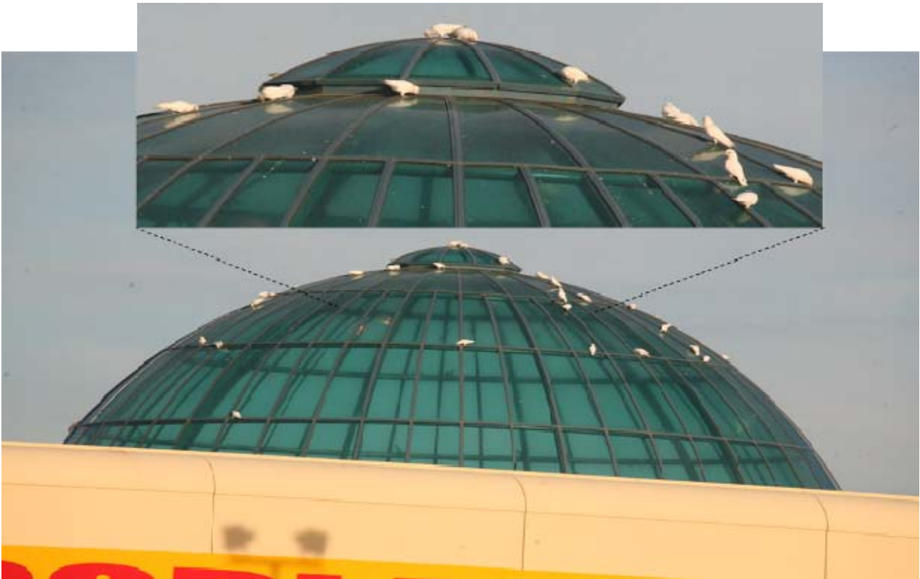
Figure 2. Glass dome on shopping centre at Seaford, with Little Corellas picking at rubber seals between the glass panels, February 2010.
