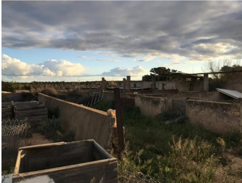
Internal wall of the eastern pens, timber fencing to complete each pen has been removed
