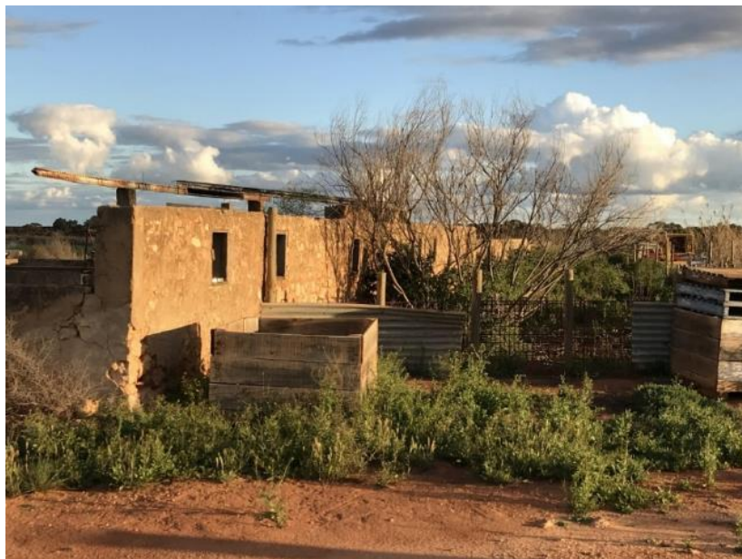
Detail of the wall western elevation, note cracking and loss of render, the fencing is a later replacement
