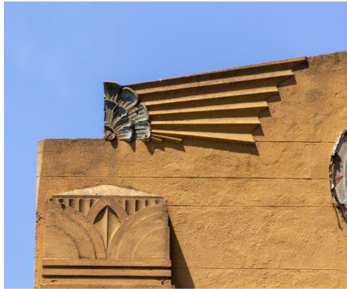
Detail showing one of the pressed cement, side acroterions with shell pattern, radiant lines and stylised decoration to top of pilaster
