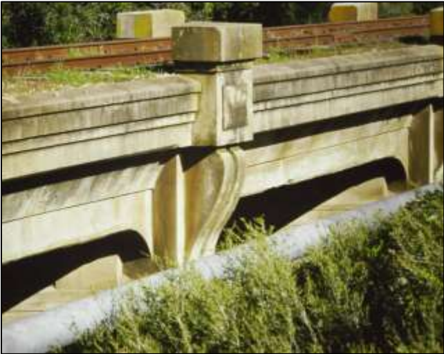
[Left] The Hindmarsh River Bridge near Victor Harbor (1908) is South Australia's first reinforced concrete girder bridge.
