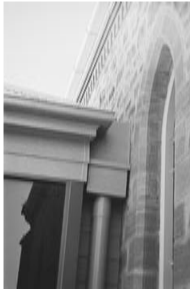
This new wall has been kept clear of the existing window opening. The new roof is separated and the junction is set back behind the downpipe and rainwater head. St Matthew's Church, Hahndorf.
