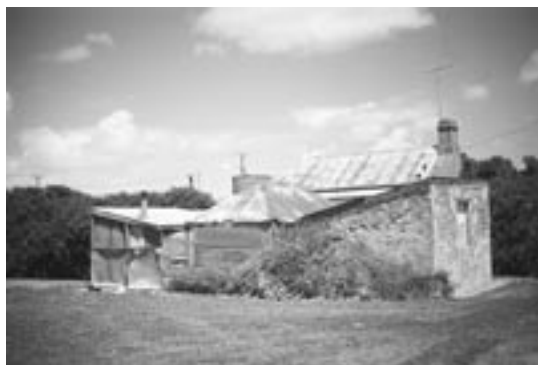
The various stone additions to this hipped roof, timber framed cottage in Robe provide clear evidence of the changing needs and aspirations of past owners.
