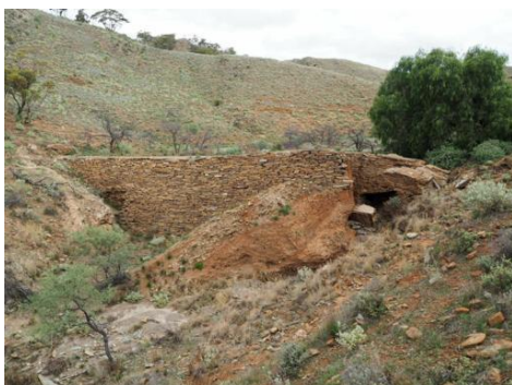
Prince Alfred Copper Mine Precinct, via Cradock [Stone-lined earth dam showing breach at west end. View is of downstream face looking south.] (DSCN P42490115 J. McCarthy)
